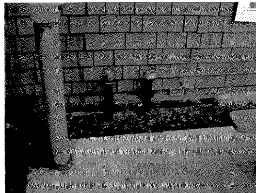
060 Fuel Oil Fill Entrance
