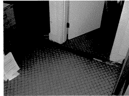
075 Electrical Wiring Along Floor
