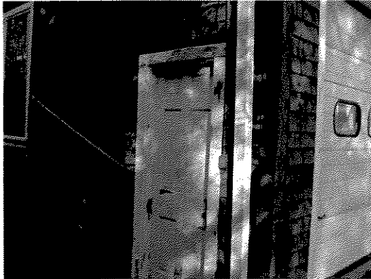
051 Peeling Wood Trim Finish
